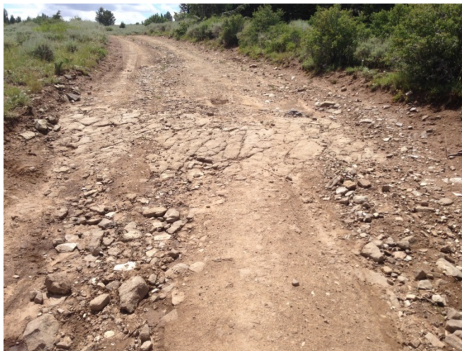
Photo 1. Improved gravel road covered with stress relief fractures.
