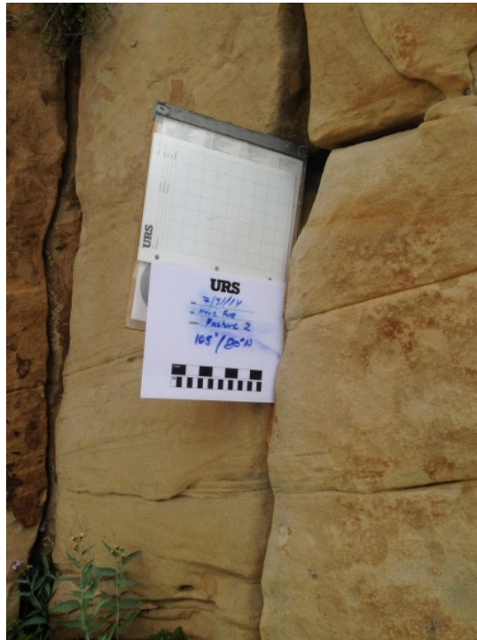
Photo 2. Fracture observed within mine portal area.
